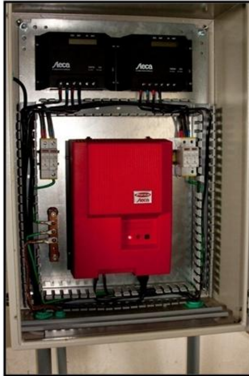
Image 8: Photovoltaic control panel 1. Photo by Kristian Bartell.
