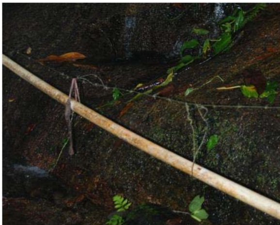
Figure 11: Exposed pipe supported by barbed wire.
