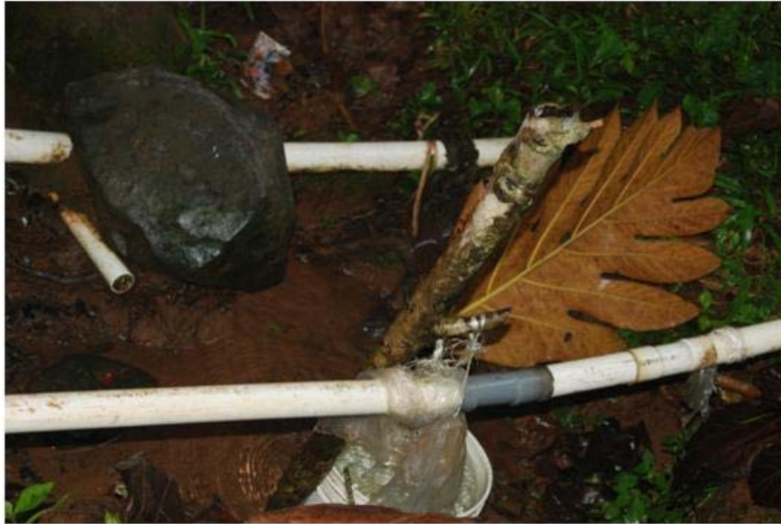
Figure 10: Depiction of leak in Calabazal’s system only taped up temporarily.
