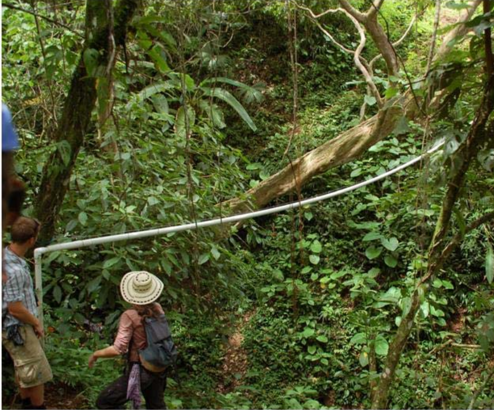
Figure 13: Depiction of pipe bridging where water pipe is encased in another PVC pipe. Additionally, showing the 90° elbow joints.
