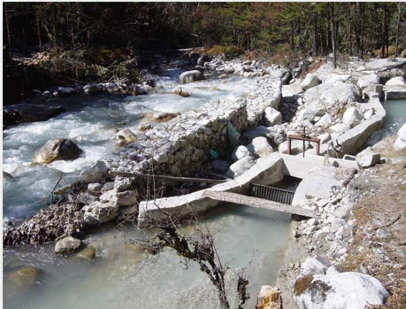
Figure 4: Example of rock diversion channel for conveying a portion of river flow Picture by Nirmal Joshi, [3]
