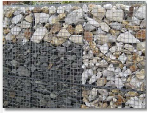
Figure 6: Example of Rock Gabion Photo by Geota [4]
