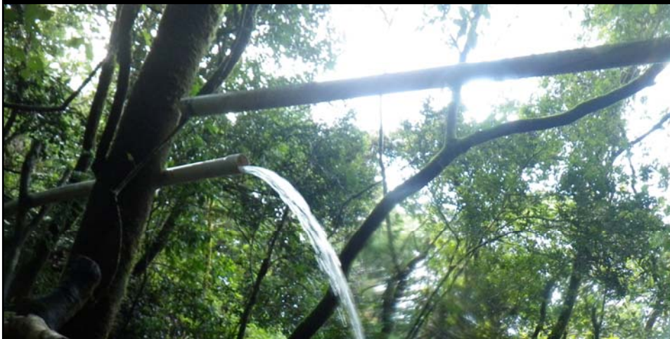
Break in pipe between Tugri and Cerro Miel
