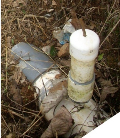
Figure16. Homemade air relief valve used on the working waterline.
