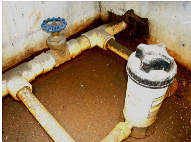
Figure 15. Chlorinator connected in parallel on the 2" waterline in Panama.
