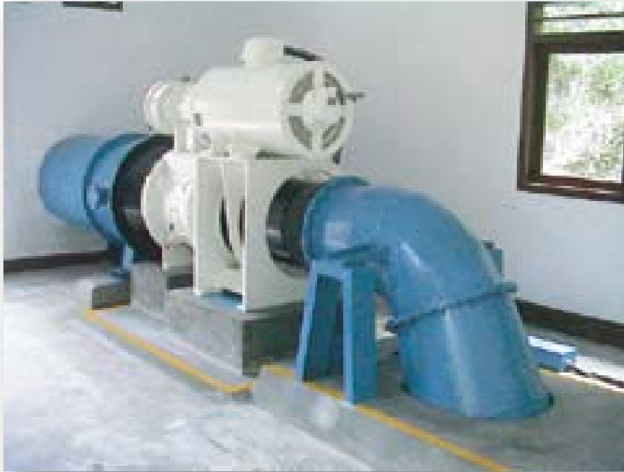
Figure 11: Toshiba Turbine - Generator [4]
