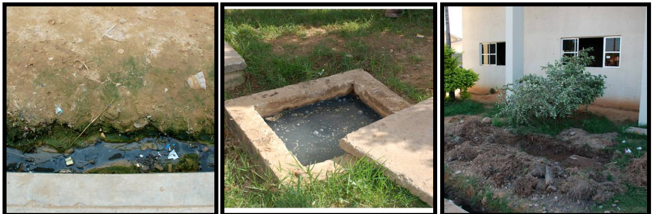
Figure 18: (L to R) Wastewater Next to Sidewalk, Full Inspection Tank, and Current Septic System
