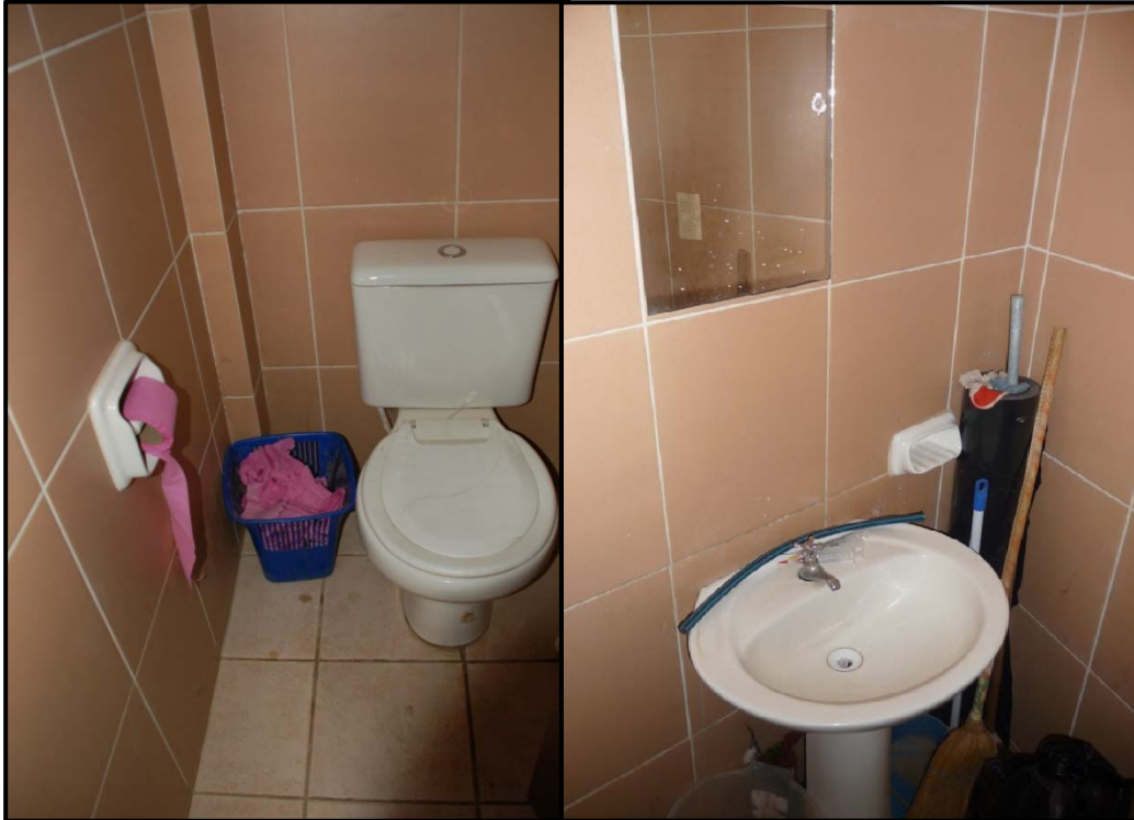
Figure 16: Bathroom Fixtures at the Police Station
