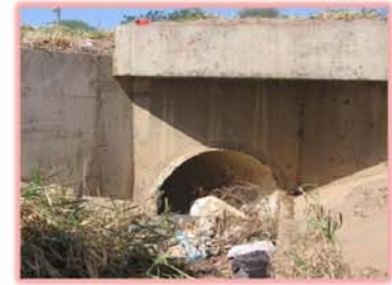
Figure 2: Culvert leading from existing canal to Doble Via. Regular cleaning of the existing and proposed canals is essential for proper functioning.
